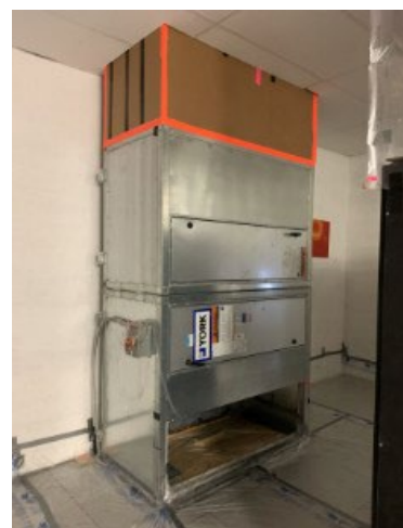
Two Computer Room Air Handlers (CRAH)
