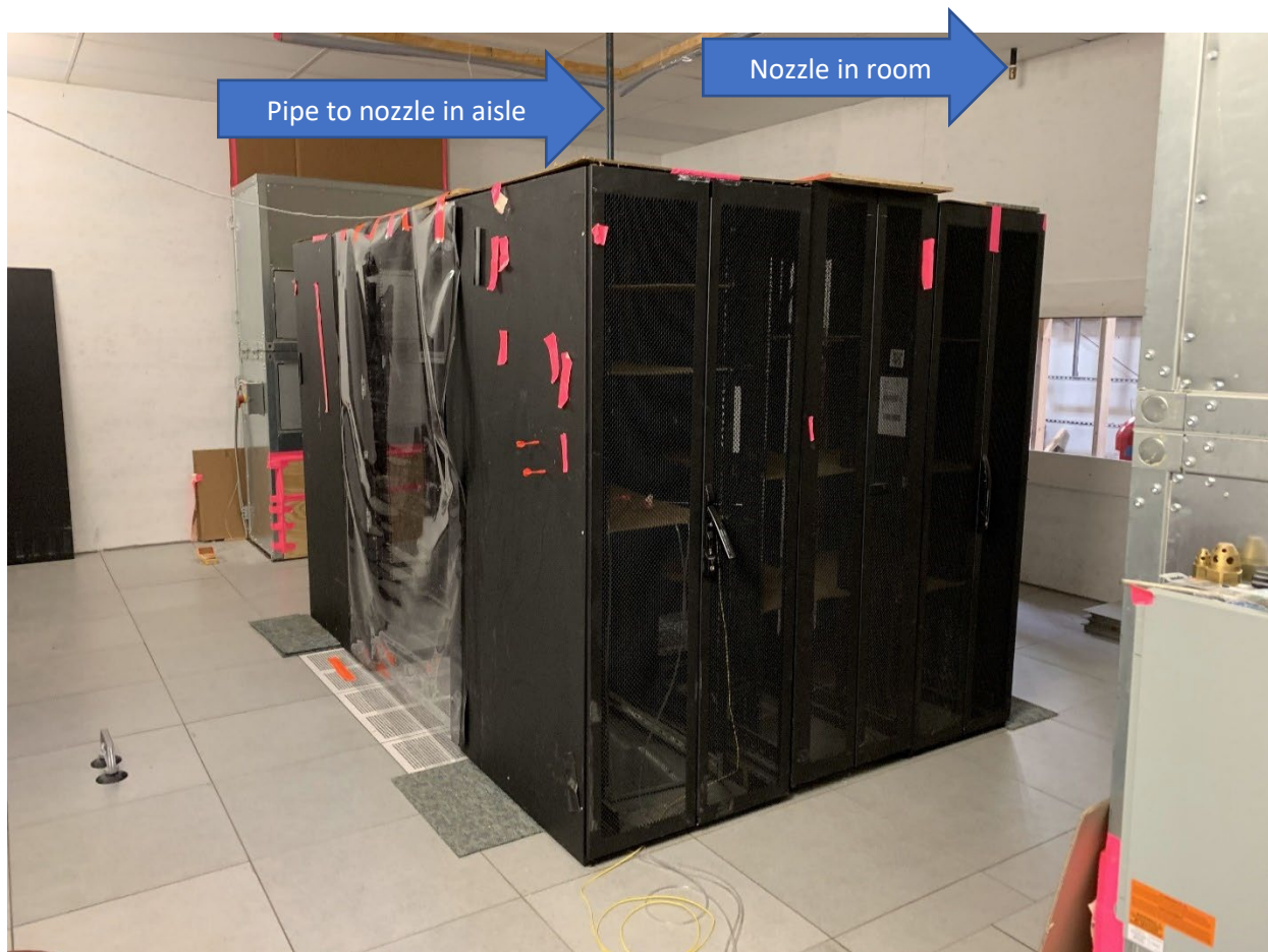
Figure 2 Photo showing the nozzle feed pipe to the containment aisle and the nozzle's location on the main room's wall. The aisle is configured as a "cold aisle."
