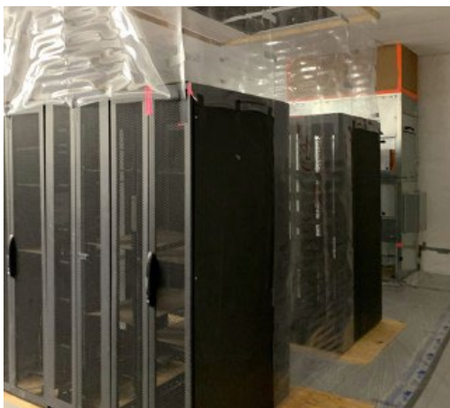
Two Rows of Server Cabinets
