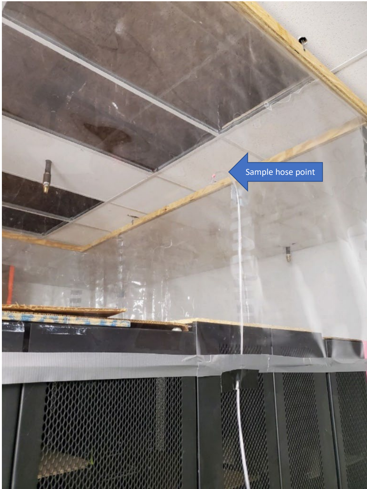
Figure 19 Nozzle inside hot aisle for tests 9, 66, 67, and 68. Concentration sample hose can be seen entering the hot aisle.
